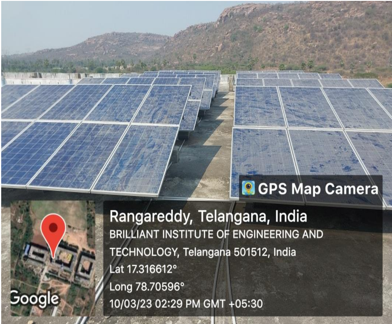
View of Solar Power plant 75 KWp.
