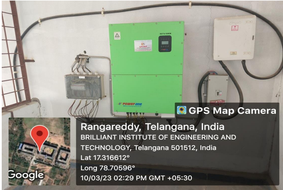
Wheeling to GRID connection
